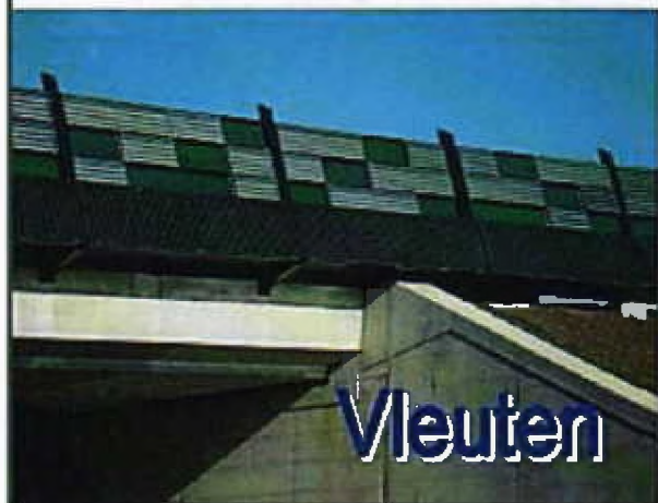
Sound absorbing noise barrier
